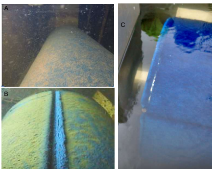
Figure 7 – Underwater photos of the TF2 unit during the trial. (A) and (B) Prior to backwashing; and (C) Following a backwash
